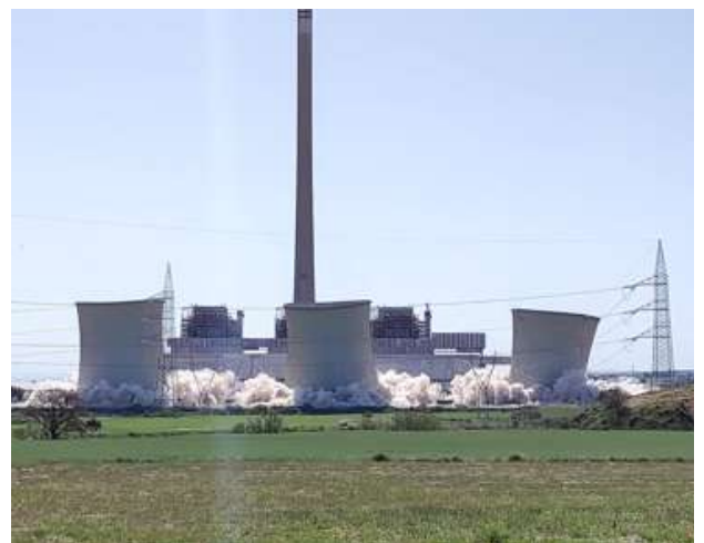
Cooling towers of the Andorra thermal power plant being demolished on 13 May 2022. Photo courtesy of Andorra City Council.
