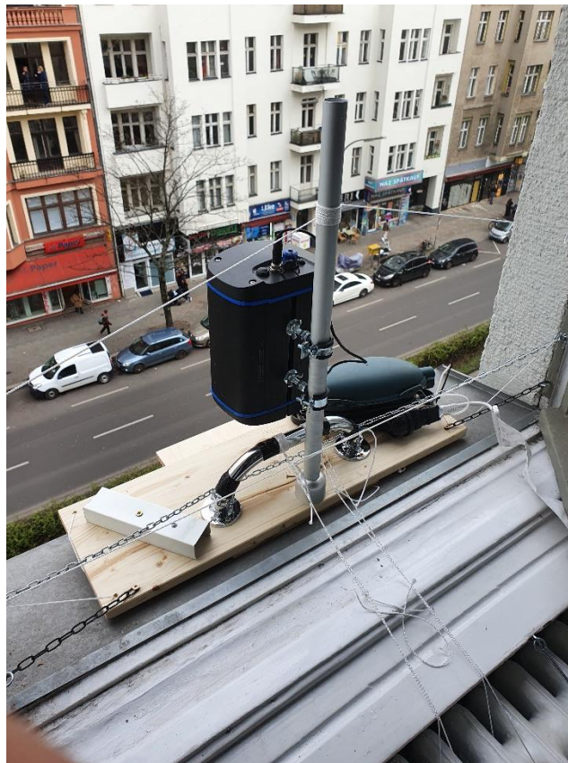
Figure S7: Zephyr system on the 4 th floor on Kottbusser Damm
