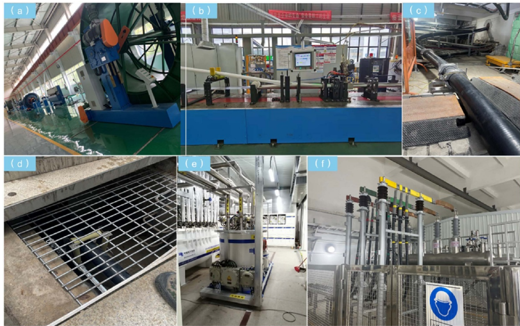
Figure 26. Landmark pictures of Shenzhen superconducting cable demonstration project. (a) Automated production line for concentric HTS cable cores. (b) Continuous welding and encapsulation production line for HTS cable core and cryogenic pipes. (c) Installed HTS cable in the cable tray. (d) Installed HTS cable in the cable trench. (e) Cryogenic refrigeration system. (f) HTS terminal in Binhe Substation.
